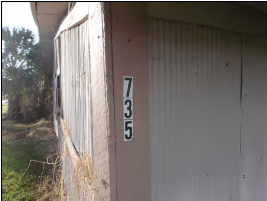
4. View of improvements at 735 5 th Avenue South, on tax parcel no. 09-34-25-0270-0000A-0006.
